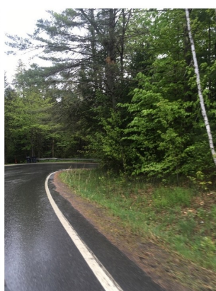
A roadside ditch, right of the white line, conveys drainage to a cross culvert which outlets west of the 111 Marshfield Rd driveway.
