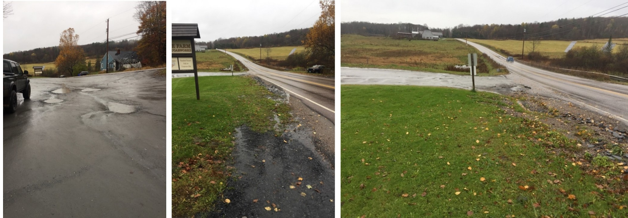
Puddles and potholes in the upper parking lot.
