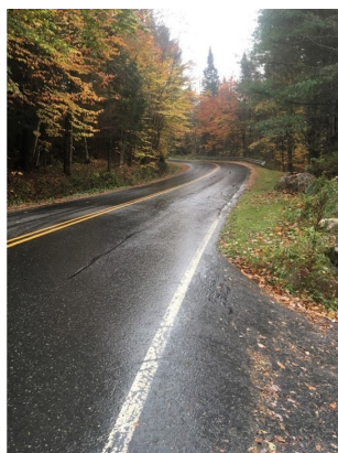
Marshfield Rd is steep and winding. Stormwater is collected in roadside ditching.
