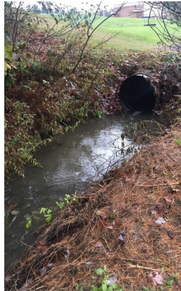
Turbid stormwater at a culvert outlet during a precipitation event.
