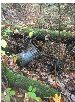
Culvert outlet located west of driveway. Stormwater is causing gully erosion at the culvert outlet.
