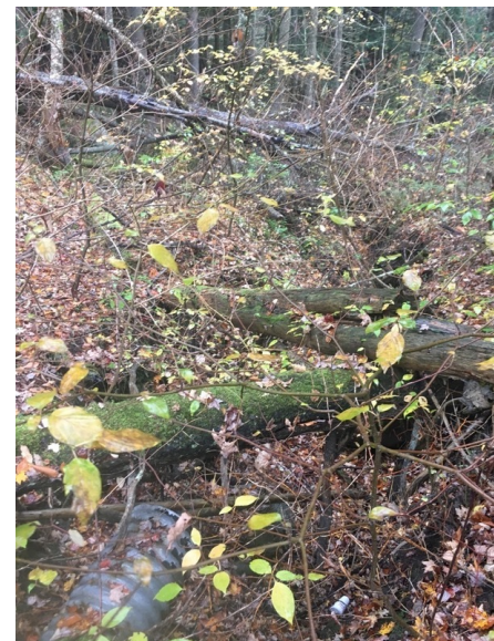
Figure A11. Gully erosion below the culvert outlet draining Marshfield Rd.
