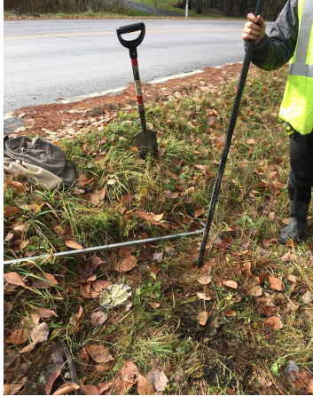
Figure A25. A hand auger and shovel were used to assess soil conditions and infiltration potential.
