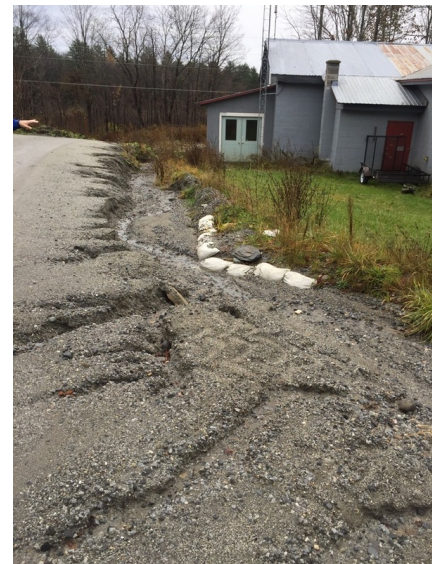
Figure B12. Sediment traps are proposed at the Town Garage and Fire Station site.
